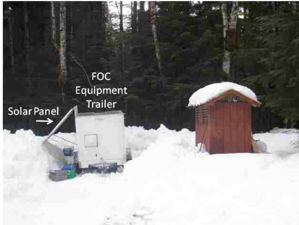
Figure 3.11 Photograph of the equipment trailer and solar panel used to power and operate the FOC. View is toward the southwest, with the Bear Creek intensive gap plot in the forest shown in the background. Partway through the deployment, the trailer was moved further away from the trees in an attempt to reduce the time during which the solar panel was shaded each day.
